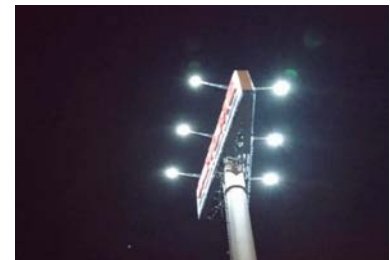
Lighting operated by solar cell Janome Thailand, Co., Ltd.
