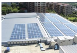
Solar power generation system
